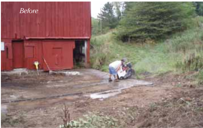
The water quality issue on Tom Kaufman's beef farm in the Town of Delhi involved an existing 25' x 48' heavy-use area concrete pad, situated at the end of the barn and base of a hill. (See photo above.) The site allowed runoff water to collect where beef cows stepped off into pasture creating a very muddy situation. A pond 30 feet away downhill from the area received the sediment-laden runoff.
