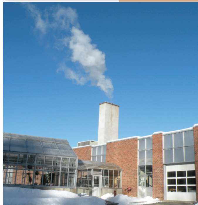
Figure 2. Even on a cold January afternoon, the wood pellet boiler at Elm Hill Elementary in Springfield, Vermont has no visible emissions (top). Across town, the Springfield High School's larger wood chip boiler system emits water vapor (bottom).
