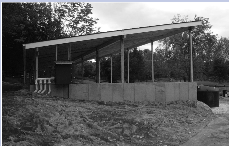
Side view of forced-air composting facility: This particular facility was constructed with four bays which would aid in the composting of approximately 200 cubic yards/month of material. The concrete, timber, and asphalt shingle structure has dimensions of 33' x 67' with a 10' roof height clearance in the front to account for the height of the front loaders.
