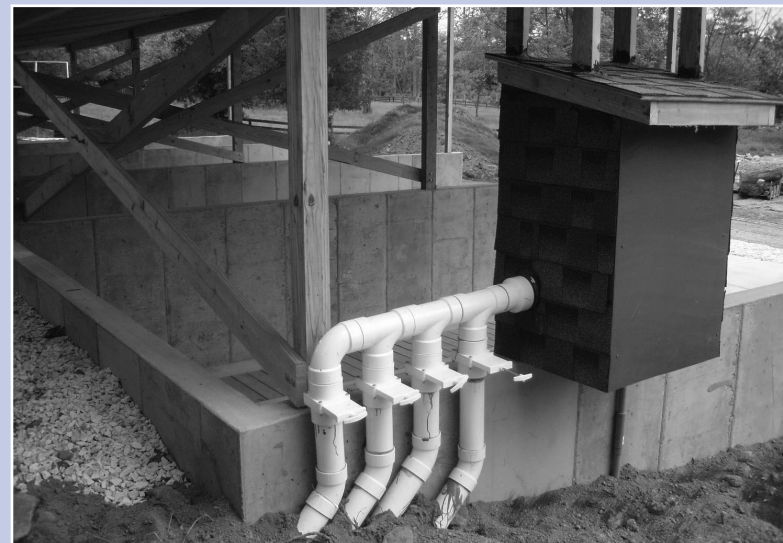
Aeration piping, gate valves and blower housing: The 1.5-hp blower operates through a cycle timer which the owner can set at 12 hour intervals. Each bay of the compost facility is supplied forced air from the blower through a network of 3" PVC pipe. Each of the bay's air inflow can be turned on and off through the 3" gate valves shown in the photo above.
